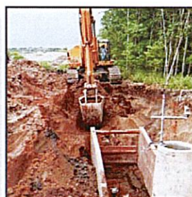
Figure 1: The capital improvement plan is used to identify, prioritize and assign funding to major capital expenditures such as land, buildings, public infrastructure and equipment.
